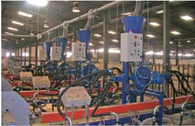
»1 Gas and coal installation
